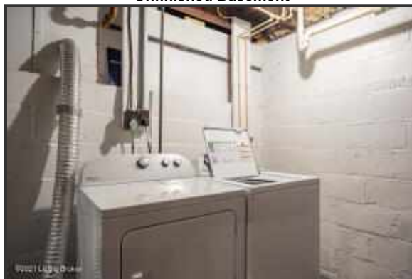
Washer and dryer hook-ups located in basement
