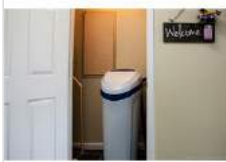
The home features a new water softener system
